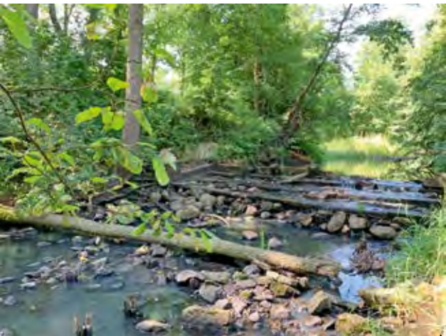
Old water threshold made from railway sleepers on the river Kamienna, Poland (WULS)
