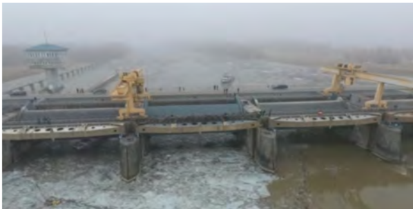
Figure 68: Kisköre dam ice passthrough
