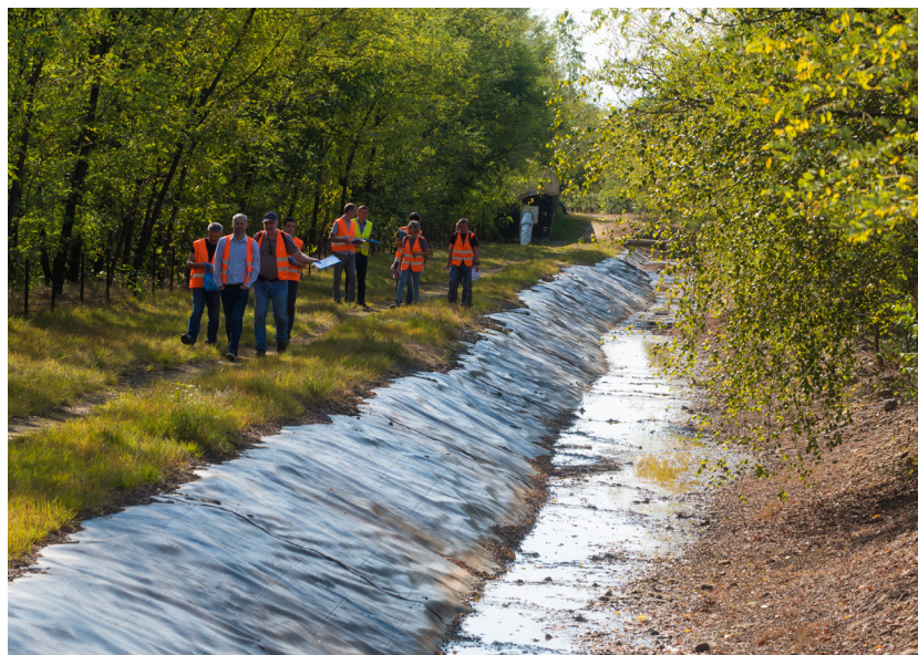
Visual check of the Aurul TMF: main drainage channel with impervious HDP screen (geo-membrane)
